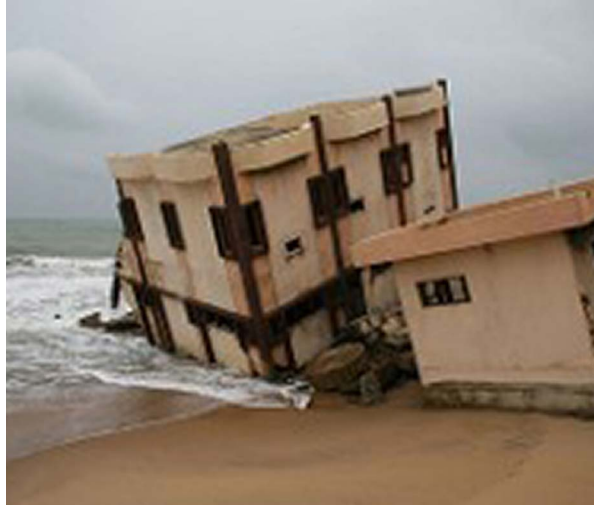
This photo of the Palm Hotel is iconic; the collapse of the Benin hotel in 2002 has been attributed to erosion, in part due to sandmining (BBC).
